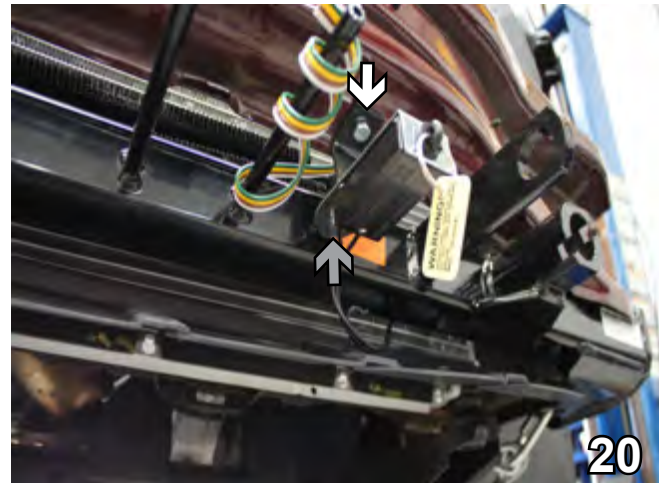
20. Optional: Using a 9/32" drill bit, drill a hole into the bottom side of the bumper centered between the electrical rod and the convenience link. Attach the bracket with 1/4-20 x 3/4" hex bolt and 1/4-20 hex nut (white arrow). Fasten the breakaway to the bracket with a 1/4-20 x 3/4" hex bolt and 1/4-20 hex nut (gray arrow).
